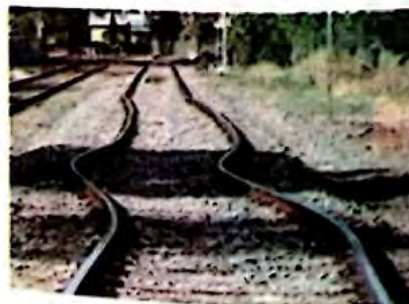
Figure 10.13 Buckled Track due to thermal expansion
